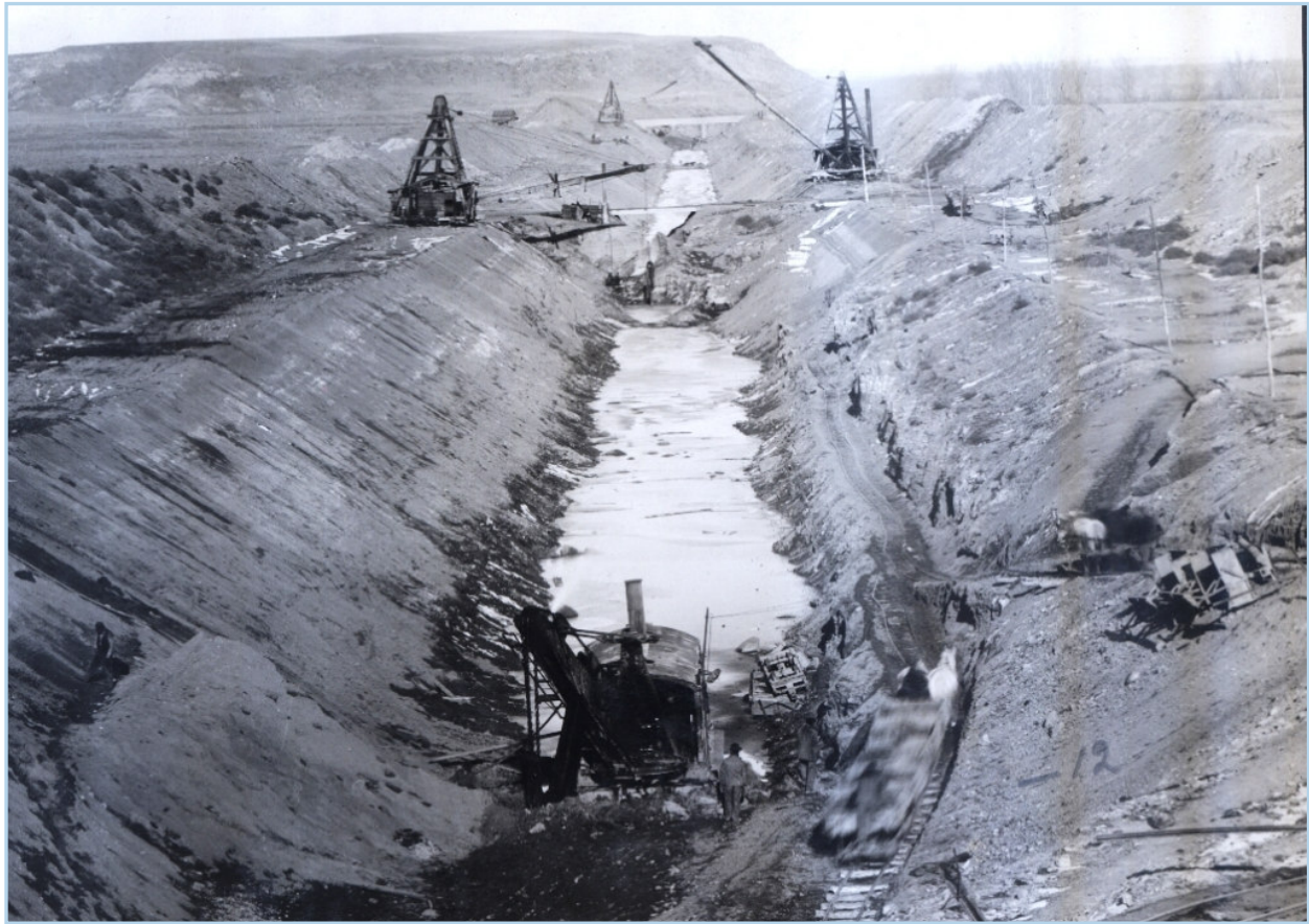
Construction of the main canal just below the intake gates in November 27, 1908
